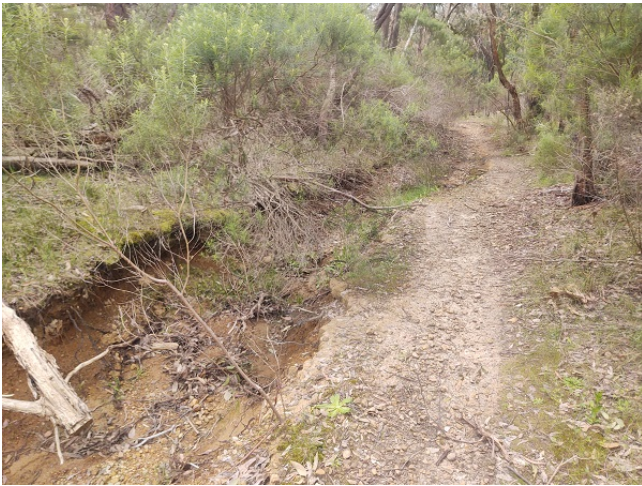
Photo 6. Soil slumping clear along the bank of a gully.
